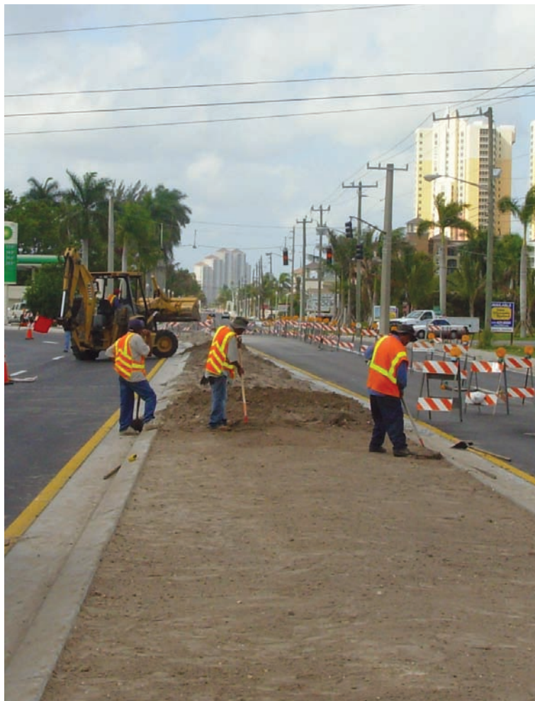
This new median under construction in Fort Myers, Florida, will limit access along State Route 80.
