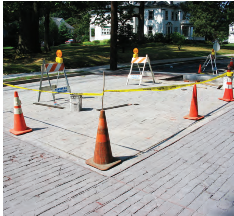
Raised intersections are being constructed on Woodland Road in Newton, Mass. to increase pedestrian safety.
